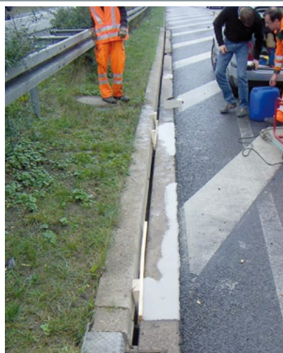
Shuttering and installation Shuttering, mix up the material, install. Wait a short period of time. Remove the shuttering.
