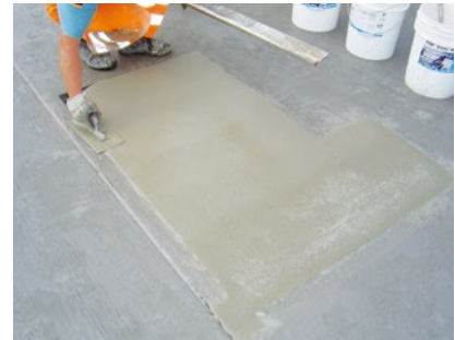
Smoothing The smoothing or removal of any excess must be done immediately. After 8 hours a compressive strength of approximately 30 N/mm 2 is reached.
