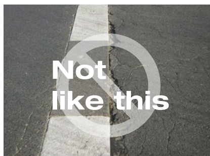
Installations in asphalt are often damaged because no joints are created.
