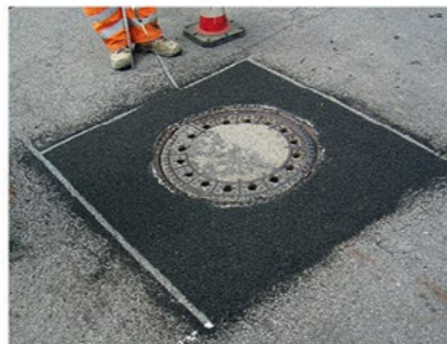
Removing the masking tape After an approx. 1 hour wait, the masking tape can be removed.
