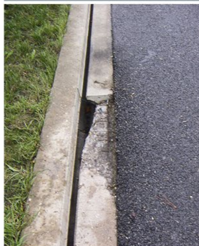
Damage to the slotted channel Concrete chipping in a slotted channel.
