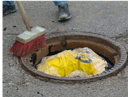
Shaft damage After restoring the destroyed mortar joint with an elastomer mortar, the road surface is normally under the height level of the manhole ring.
