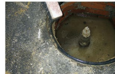
Cleaning After opening the manhole cover, clean the supporting edge of any gross contamination.
