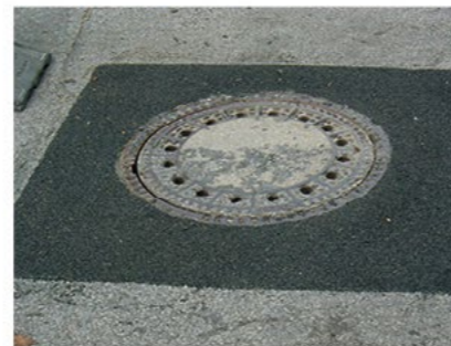
Finished levelling layer Finally the excess material used for sprinkling is swept off. Traffic can then be released.
