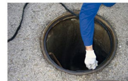
Install the formwork On the inside edge of the cover support, apply TOK®-Band SK 25 x 8 mm with approximately 3-4 mm protrusion.
