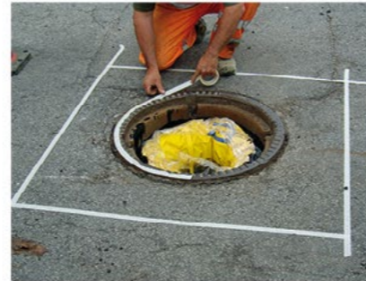
Mask the manhole ring The manhole frame should also be masked off.
