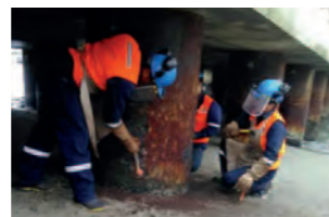
Heavy corrosion on piers
